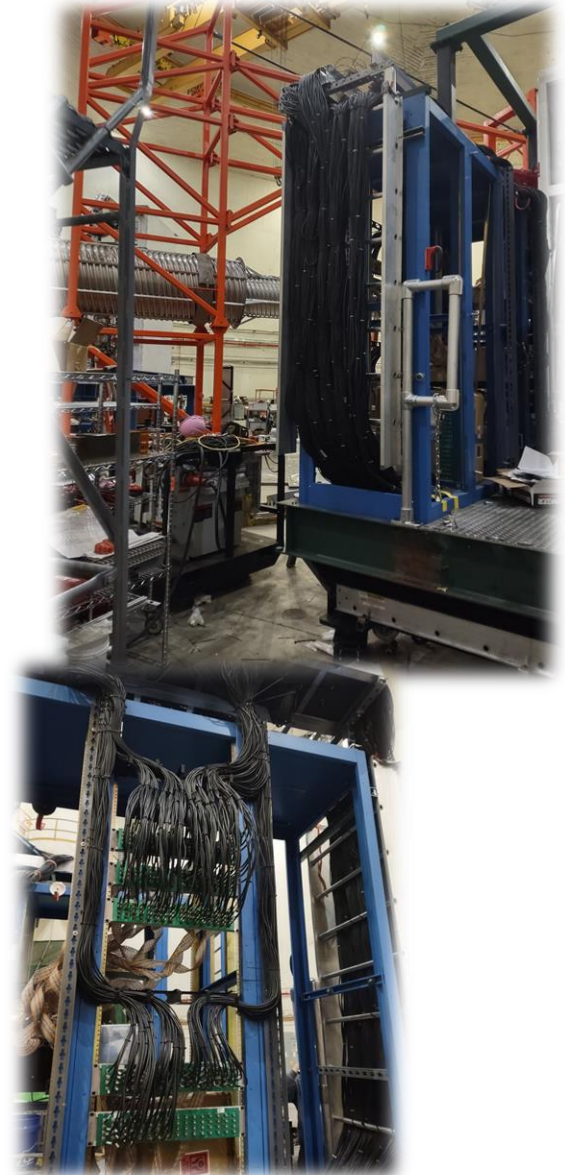
Cable trays on the platform
