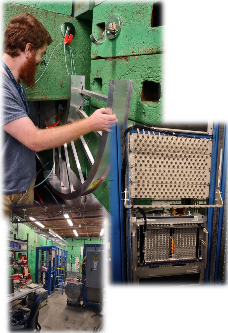
Cable trays in the SBS bunker (DAQ)
