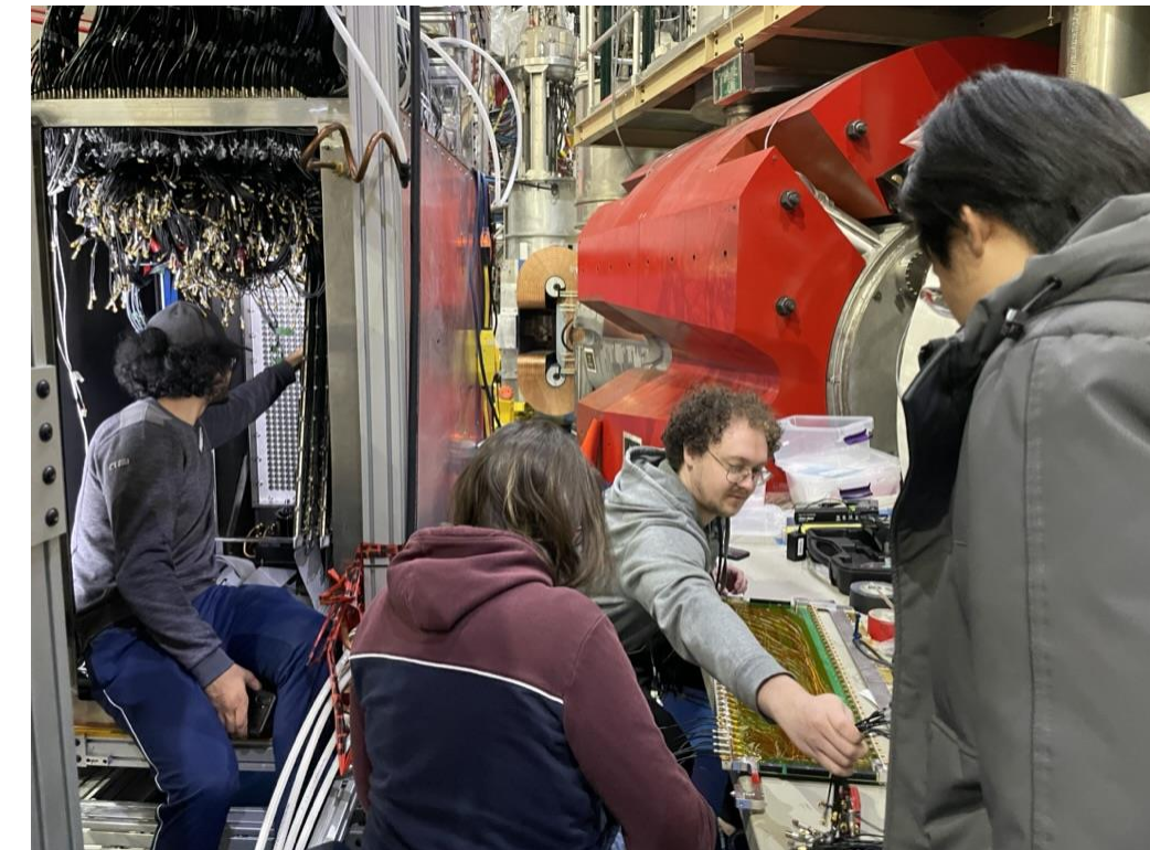
Checking the application of optical grease (top) and reconnecting the distribution boards (bottom) during 2023-2024 Winter SAD
