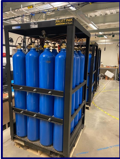
HP Gas cylinders
