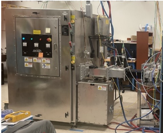
AMTek Commercial 75 kW CW magnetron supply with JLab modified controls
