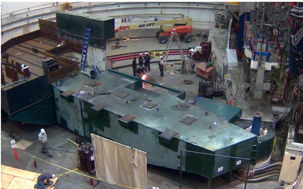
Hall C SHMS Support Structure, self supporting.
