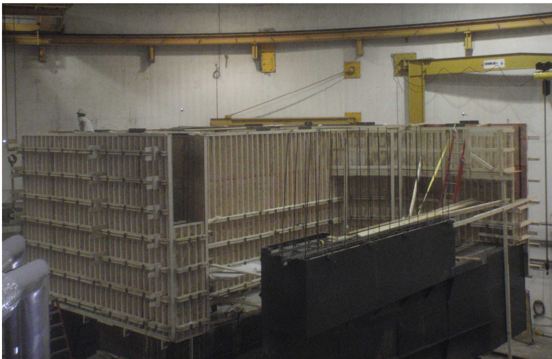
View of the forms for the SHMS shield house showing the detector site.
