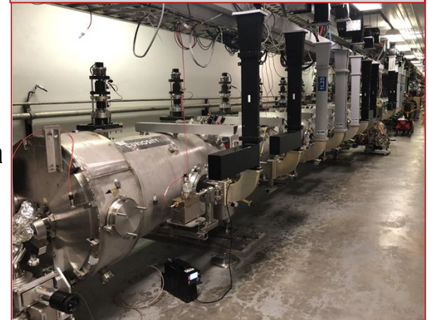
Refurbished C100 In North Linac
