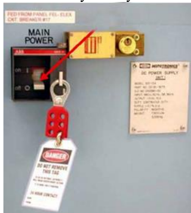
Figure 3 – Main Circuit Breaker and Locking Systems
