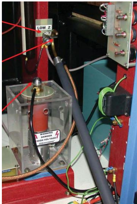
Figure 4 - Location of Lo-Z grounding point in CPS
