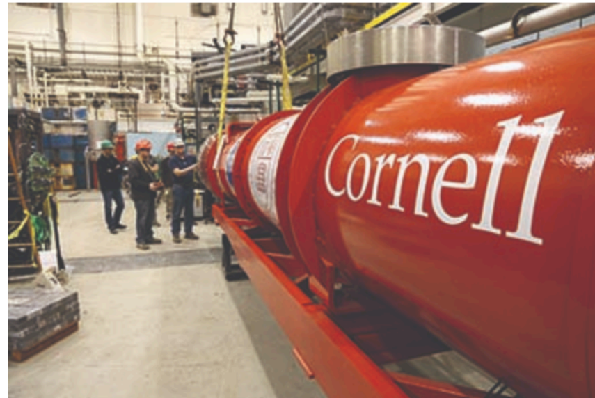
The main linac cryomodule
