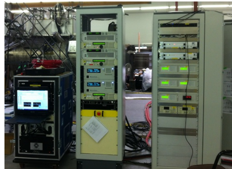
FIGURE 6. Quench protection DAQ, instrumentation and power supply control.
